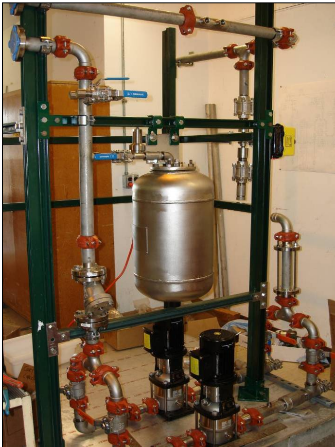
Figure 3. Prototype de-ionized cooling water circuit for cooling NSLS-II magnets and absorbers, assembled at NSLS.
