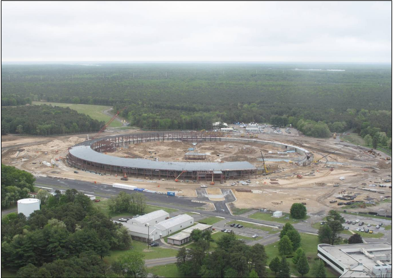
The Ring Building takes shape, with erection of structural steel progressing rapidly in this photo taken April 30.
