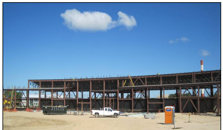
Figure 7. Structural steel and roof decking for Ring Building pentant 1, RF bldg, and service bldg 1 are near completion.
