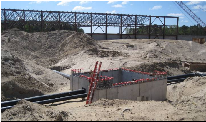
Figure 8. Steam manhole 47D being installed as part of underground utility work in the Ring Building courtyard.
