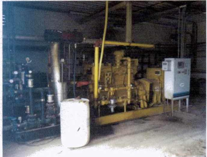
Digester Engine and Generator
