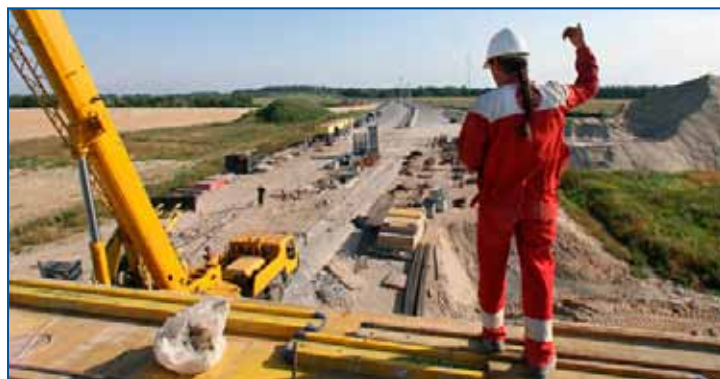
The Recovery Act is helping to stimulate construction and jobs in communities across the nation.
