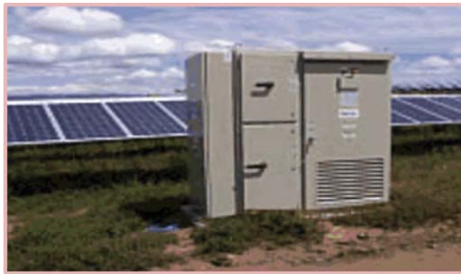
Figure 2- 11 Solar Ground-mount Grid System
