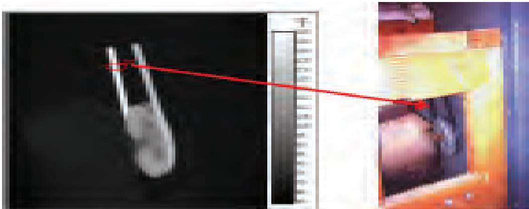
Figure 6.2.3. Temperature is used in defining belt problems. Figure shows a belt temperature of 149°F, and ambient temperature of 67°F for a difference of 82°F. The difference should be trended over time to determine slippage that would be indicated by a higher temperature difference.
