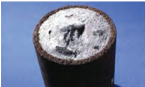
Figure 9.2.8. Boiler tube – scale deposit
