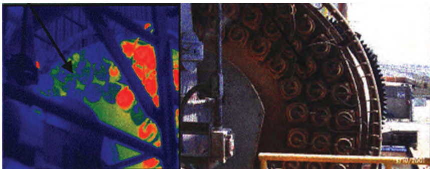
Figure 6.2.9. Inoperable steam heaters seen by cooler blue areas when compared to the operating heaters warmer red or orange colors.
