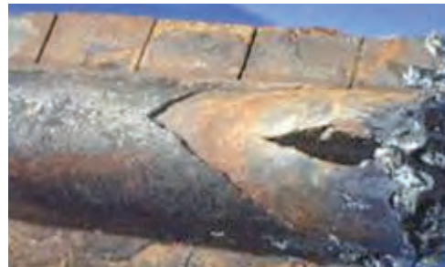
Figure 9.2.9. Boiler tube – failure (rupture)
