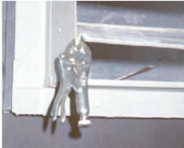
Figure 9.7.2. Damper quick fix – not recommended
