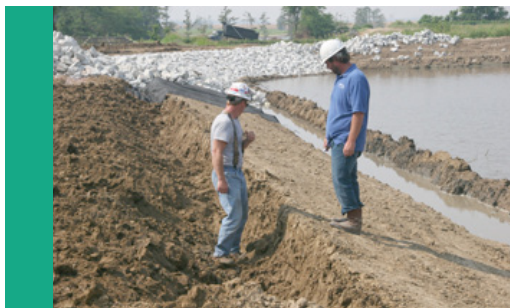
Brian Gawf (right), NRCS construction inspector, looks at a trench created to hold rocks on the levee around a sewage treatment facility lagoon.
