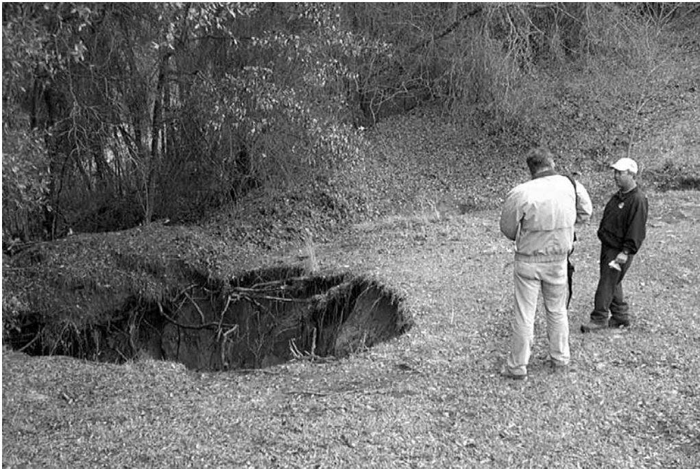
Evaluating erosion problem
