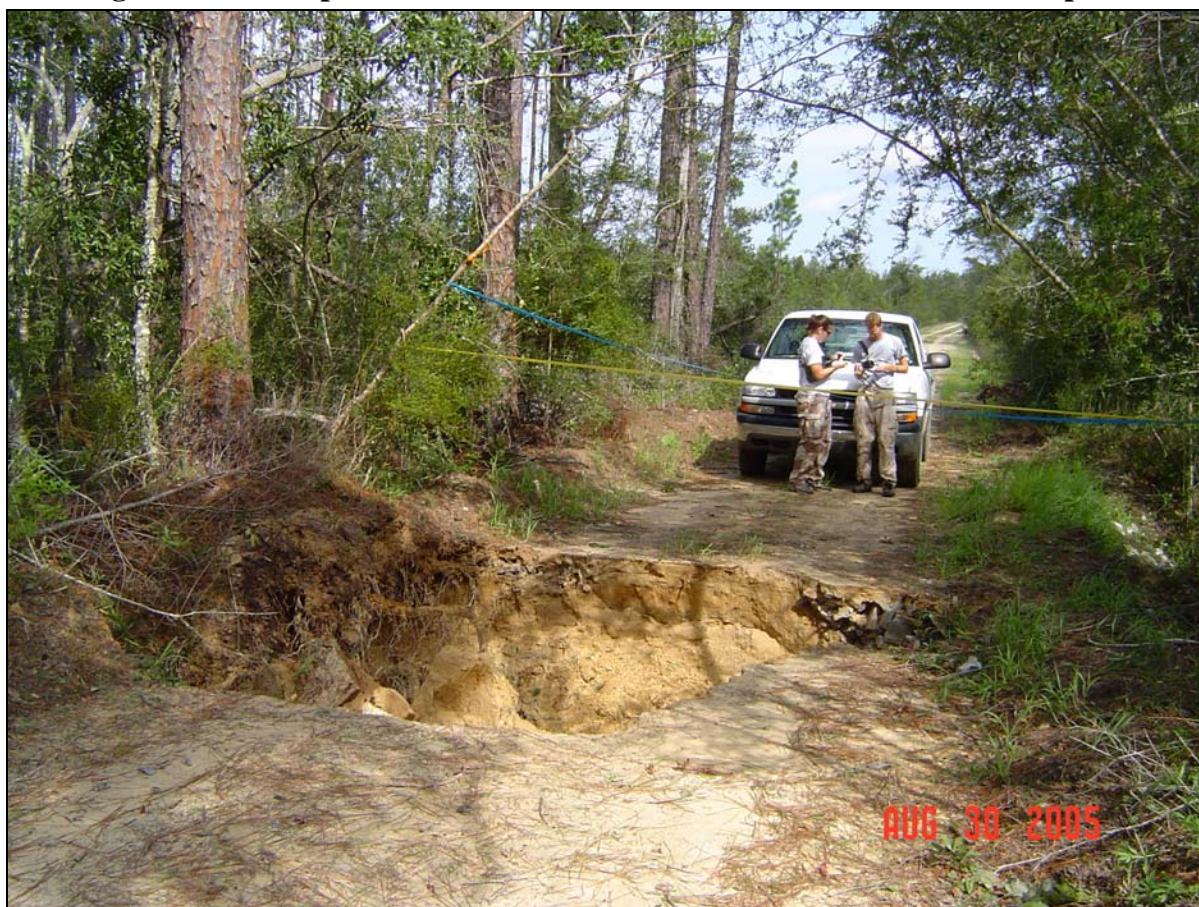
Figure 17: Example of Dirt Road Issues within the Perdido River Floodplain
