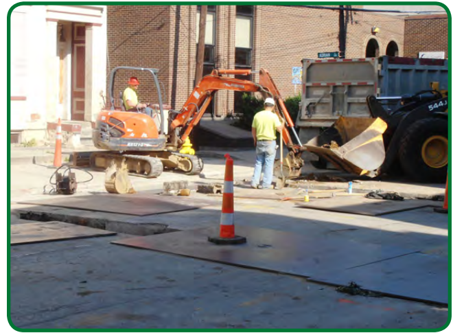
Greater Cincinnati Works does infrastructure work to prepare for the Cincinnati Streetcar. Image courtesy of the city of Cincinnati.
