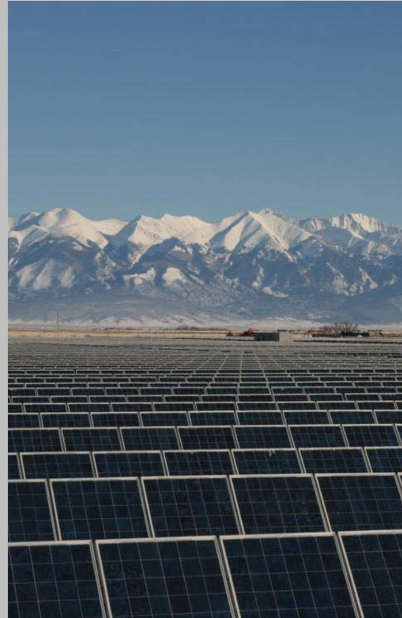
8.22-megawatt Alamosa, Colo., PV solar plant
