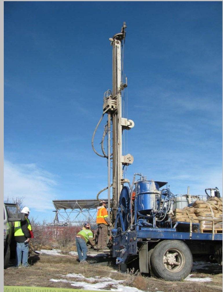
Drilling rig on South Table Mountain, testing for installation of geothermal heat pump showcase system at NREL.
