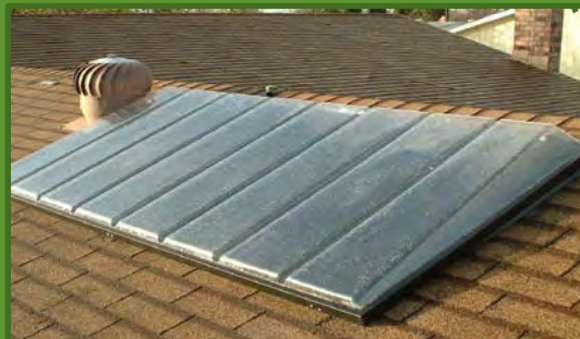
Polymer Solar Water Heaters
