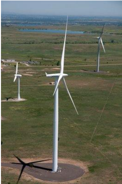
The Siemens 2.3 MW turbine at NREL is among the largest land-based turbines deployed in the United States
