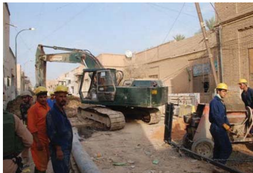
Iraqi workers on the site of the $1.8 million USACE-managed sewer project in the Adhamiya neighborhood of Baghdad. (USACE photo)
