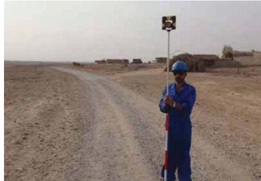
An Iraqi helps survey one of the rural roads in Tameem province designated for resurfacing through the “Village to Market” program. (USACE photo)
