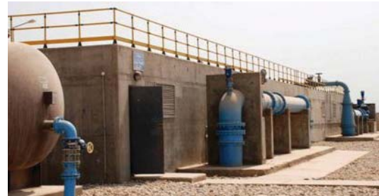
The $65 million Sadr City R3 Water Treatment Plant is designed to provide more than 500,000 Sadr City residents with potable water. (USACE photo)
