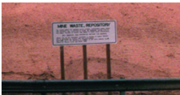
A guardrail barrier (weathering steel) was installed at the base of the American Fork repository to prevent access by motorized vehicles and disturbance to the repository cover materials and vegetation.
