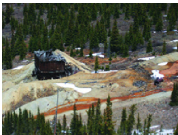
Cleanup of the Pennsylvania Mine on the White River National Forest. This is one of the abandoned mines in the Peru Creek Basin.
