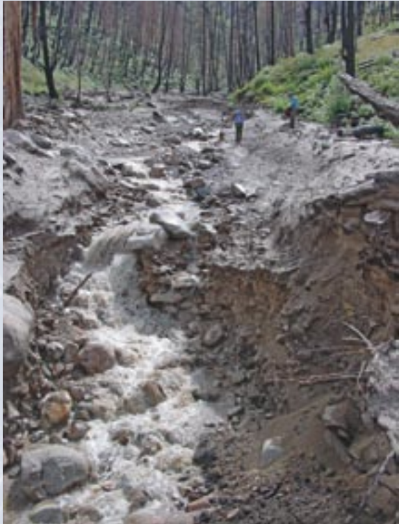
Erosion at Lake Creek, a tributary of the Boise River, ID, following fire. August 2004.
