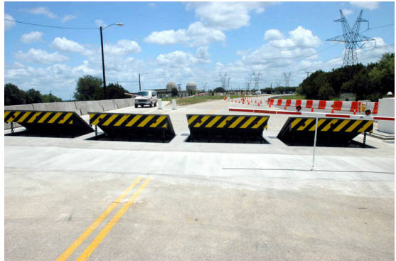
Changes to the DBT have warranted an increase in physical security, including enhancements to vehicle barriers.
