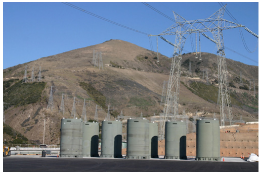
Independent spent fuel storage installations are used to safely store spent fuel.
