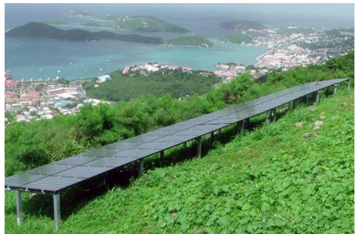
Figure 3. 10 kW PV system installed on St. Thomas, U.S. Virgin Islands PIX 19568
