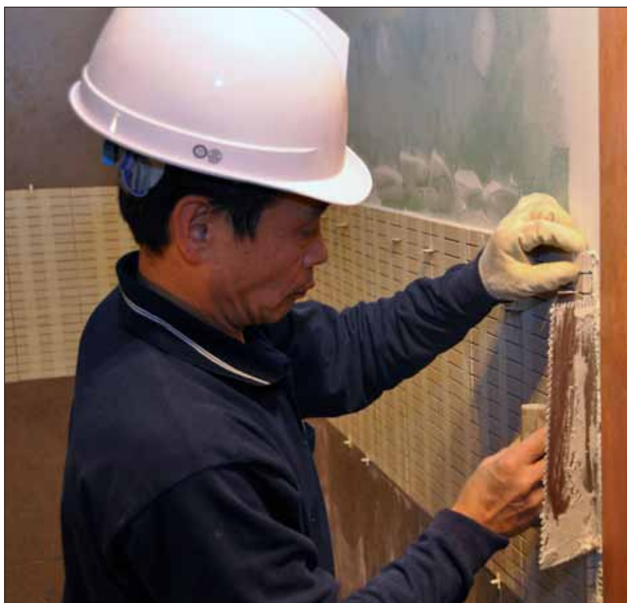
A contractor working with the 51st Civil Engineer Squadron applies wall mounts in the newly built enlisted club, Jan. 11, 2012, at Osan Air Base, Republic of Korea. (U.S. Air Force photo by Airman 1st Class Michael Battles)
