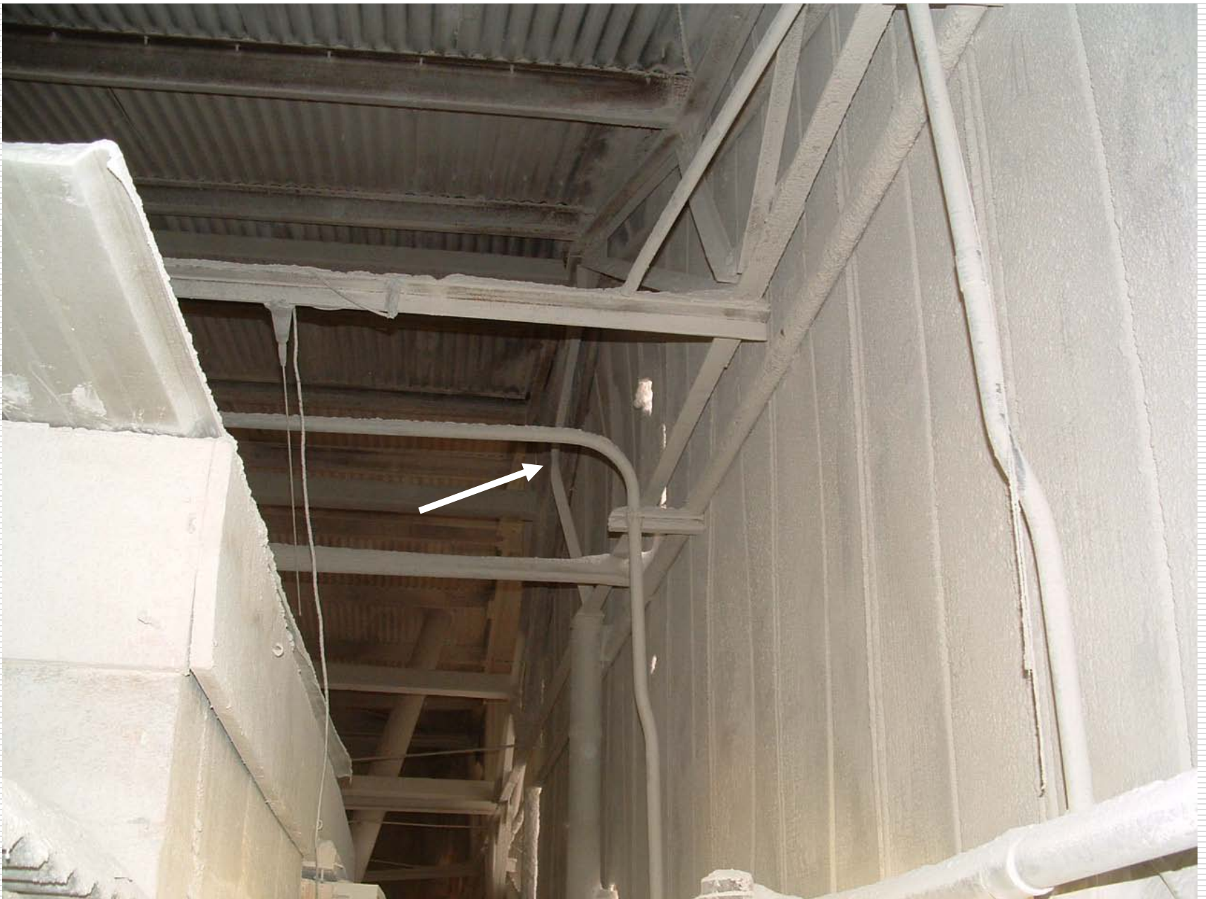
Buckled Vertical Roof Truss Member
