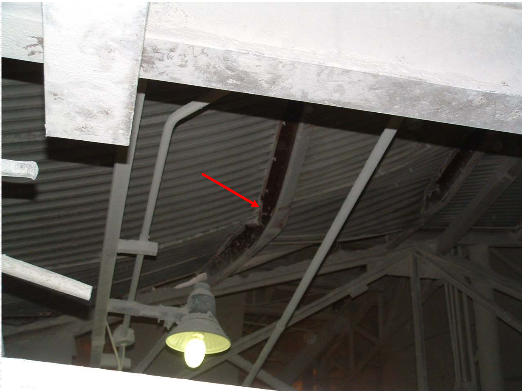
Collapsing Roof Support Purlins
