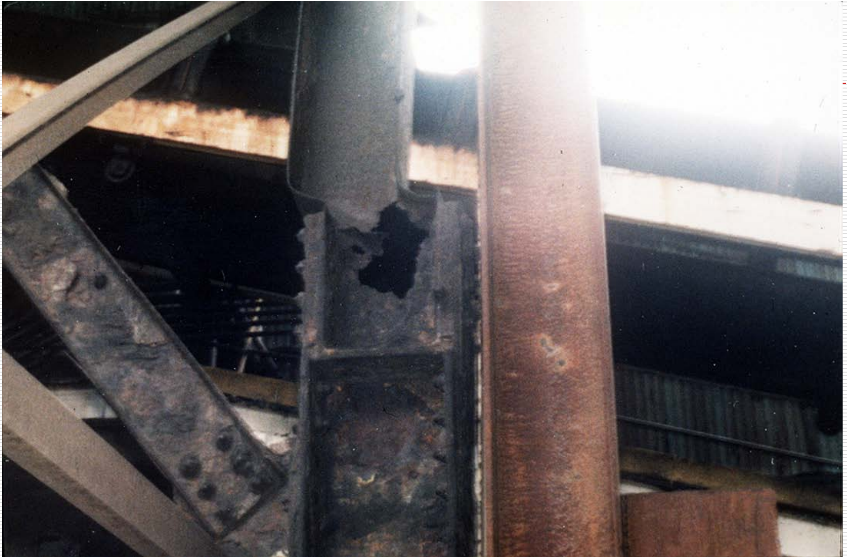
Buckled column flanges @ web corrosion hole 29
