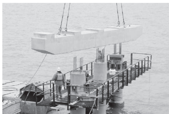
Top: The replacement of a bridge superstructure is shown. Bottom: The placement of a precast bent cap is shown.
