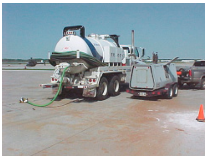
A multipurpose treatment system in use at CAAF.
