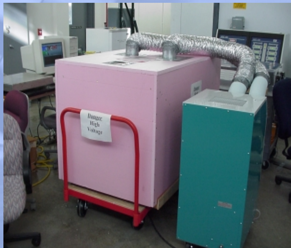
Battery pack in an insulated box with air cooling
