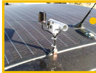
Rooftop pyranometer & RTD
