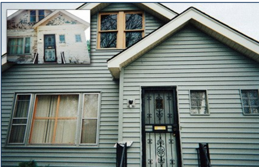
An AHP Homeownership set-aside grant was used for the rehabilitation of an owner-occupied home in Detroit. (Before inset upper left.)
