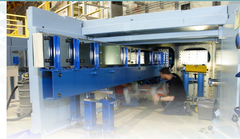
NCNR technical staff members Dan Adler and Mike Rinehart perform installation work on the new, advanced neutron guides as part of the NCNR Expansion Project. This particular guide will provide a very high flux of neutrons for experiments performed by the Physical Measurement Laboratory Neutron Physics group
