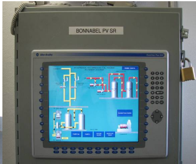
Figure 8: Allen Bradley programmable automated controller that allows remote operation of equipment from the safe room.
