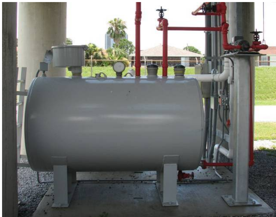
Figure 9: Bonnabel safe room (1) fuel tank, (2) pump and motor would be elevated and secured to protect from flooding.
