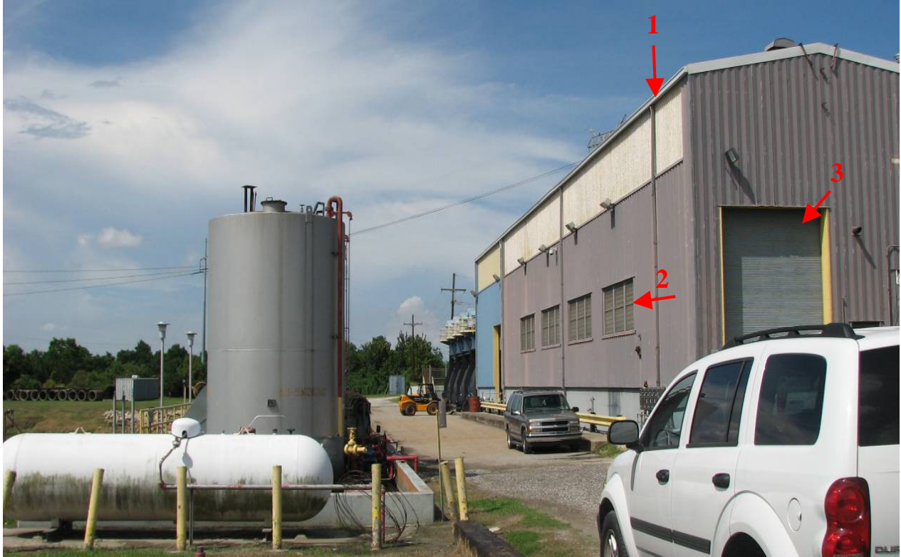
Figure 4: Features of Planters pump station proposed for stormproofing to resist wind speeds up to 140 mph: (1) roof, (2) window, and (3) coiling door.
