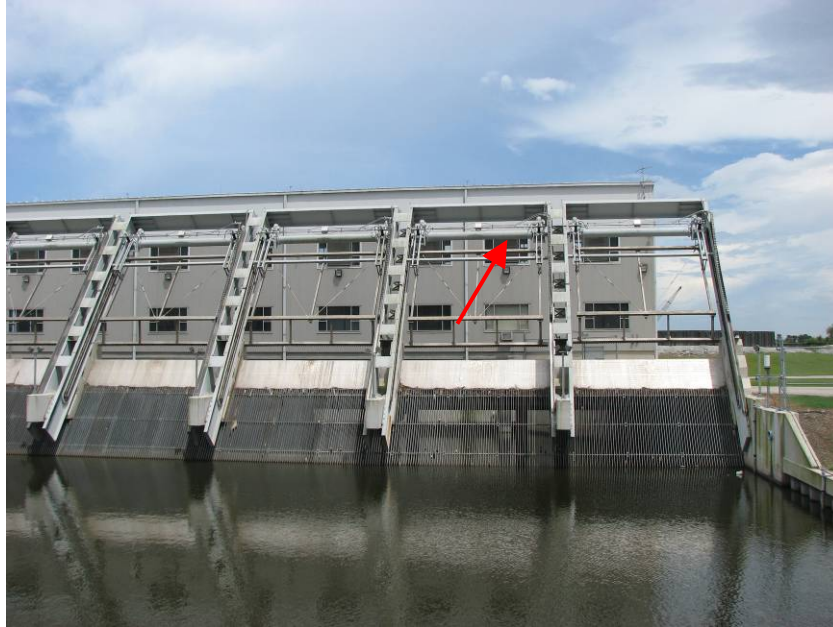
Figure 3: Climber screens at Whitney Barataria that catch debris and remove trash from pump screens.
