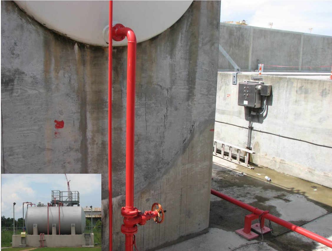
Figure 6: Bulk fuel storage tank and fuel system containment structure.
