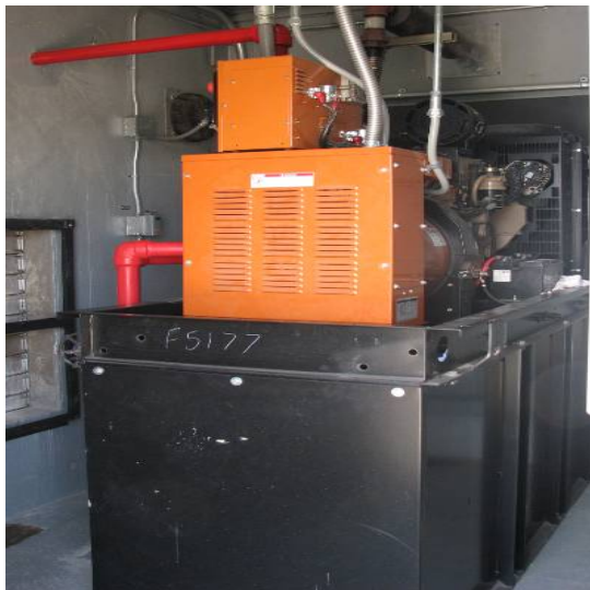
Figure 7: Bonnabel safe room generator
