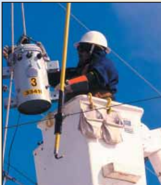
A lineman repairs damage following a winter storm in Texas. Rural telecommunications and electric cooperatives throughout the nation look to USDA for much of their financing needs. USDA photo by Dan Campbell
