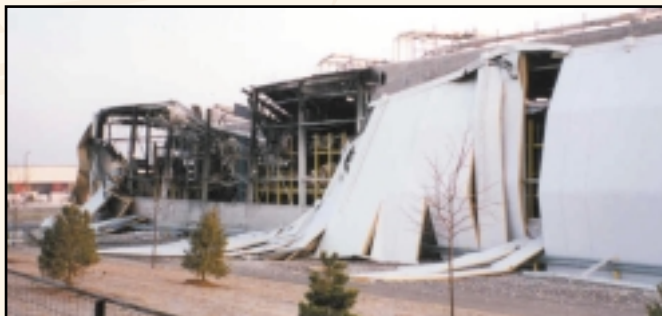
The pilot was killed and heavy damage was done to this Foremost Farms USA milk bottling plant in DePere, Wis., when a small business jet crashed into it. PHOTO COURTESY FOREMOST FARMS USA.
