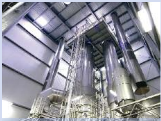
A $62-million renovation project at its Ovid dairy plant resulted in Michigan Milk Producers Association (MMPA) winning the 2010 Plant of the Year award from Dairy Foods magazine. Photo courtesy MMPA
