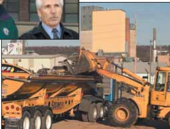
Debris is cleared following a fire at AMPI's butter plant in New Ulm, Minn. Above, Minnesota Governor Tim Pawlenty (left) and AMPI General Manager Mark Furth survey the damaged plant, which will be rebuilt in New Ulm this spring. Photos courtesy AMPI
