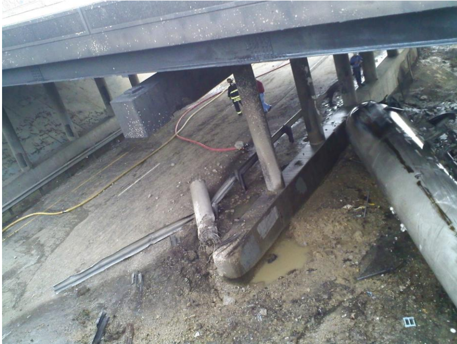
Figure 7. Displaced bridge pier column struck by cargo tank semitrailer. (Source: Indiana State Police.)
