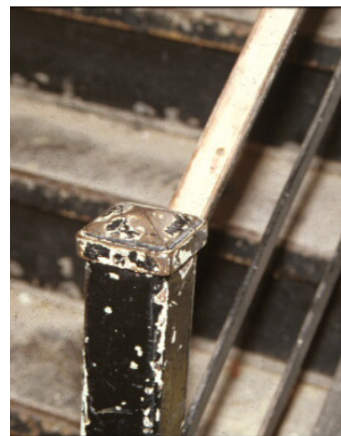
FIGURE 12.5 A metal railing before abatement.
