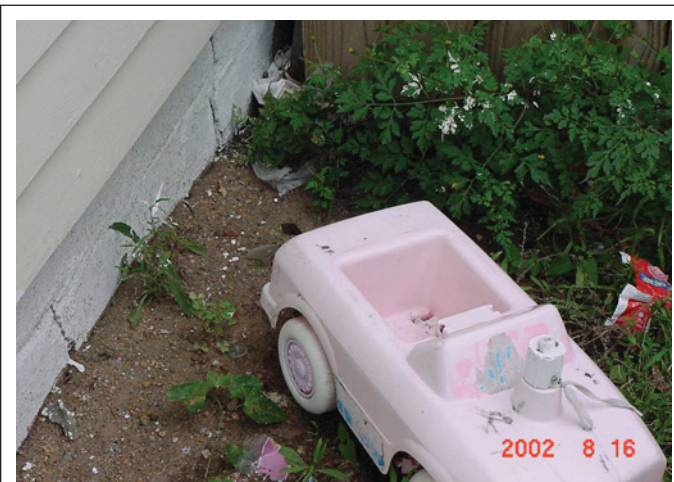
FIGURE 5.9 Soil lead hazard at dripline
