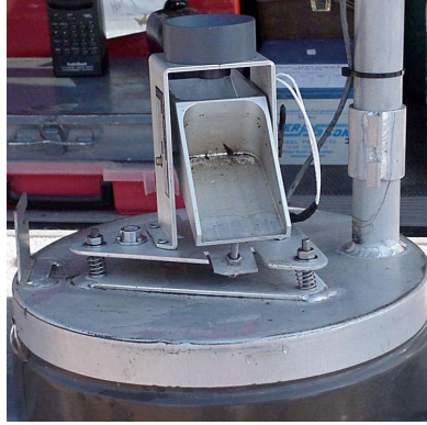
Figure F- 9. Dirty tipping bucket, side view.
