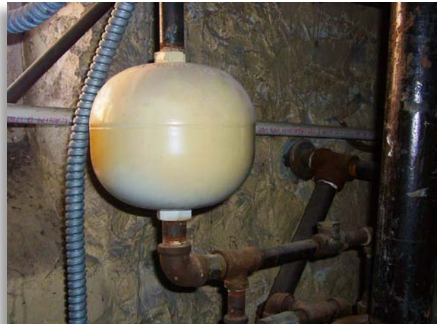
This retarding chamber attached to the wet-pipe sprinkler system reduces the likelihood of false alarms caused by water surges.
