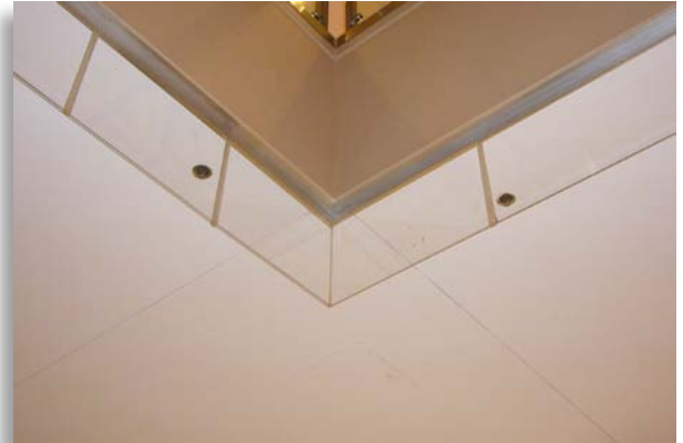
This vertical opening in this shopping mall is protected by closely spaced sprinklers and a limited combustible draft stop.
