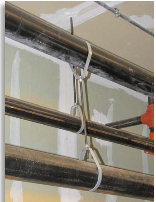
This pipe should be suspended from the structure, not another pipe.
