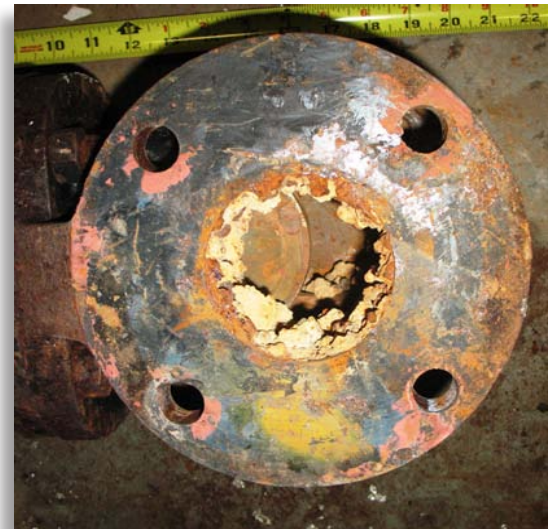
The condition of this valve assembly in the domestic service line suggests the fire protection service should be checked. Photo courtesy of Bryan Blake.
