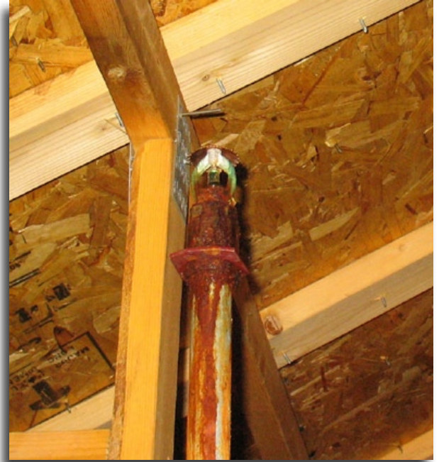
Photo courtesy of Freedom Fire Protection, Longmont, Colorado. This corroded sprinkler was one part of a larger system failure.
