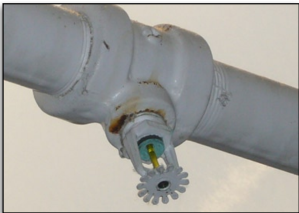
This sprinkler above a public swimming pool shows signs of corrosion.
