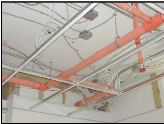
Lay-in ceiling tiles will provide an approved thermal barrier for CPVC.
