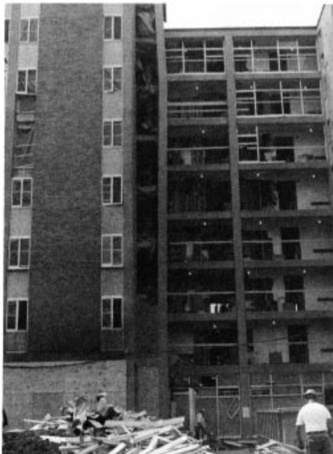
Figure 3. Back of Gross Towers after Accident
