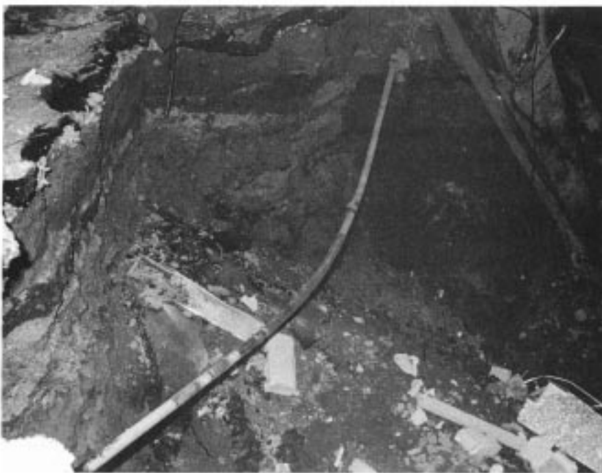
Figure 4. Gas Service Line after Explosion
