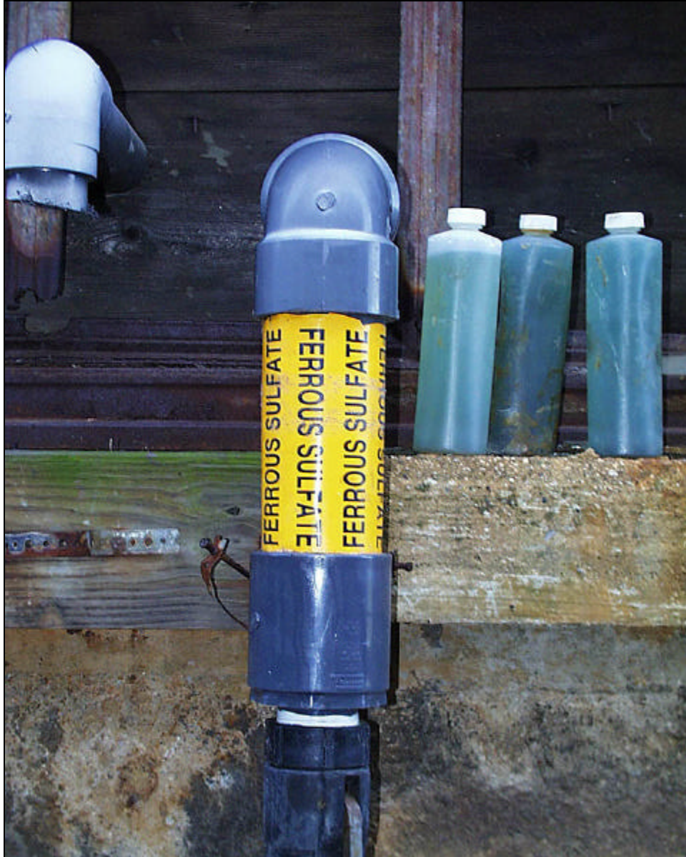
Figure 2. Close-up view of ferrous sulfate transfer coupler
