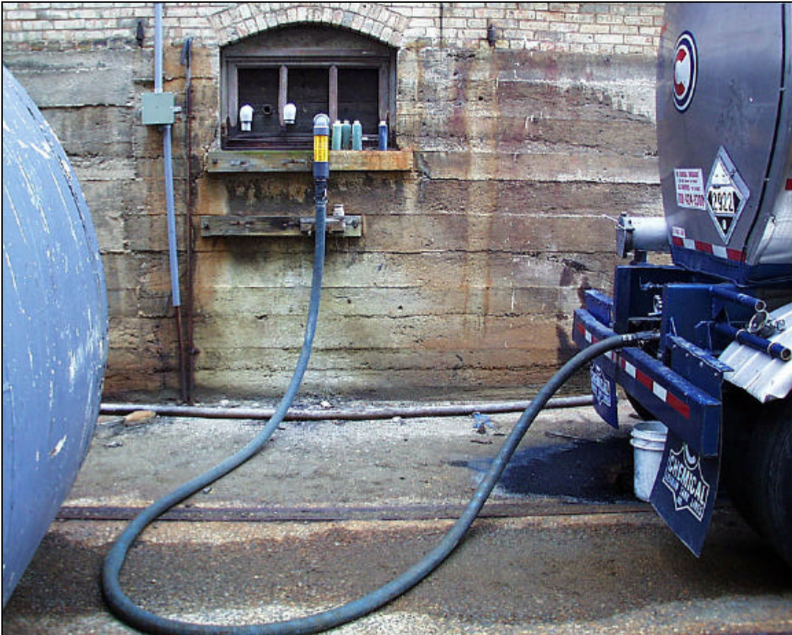
Figure 1. Postaccident view of the cargo tank (right) with transfer hose attached to the ferrous sulfate transfer coupler. The two pipes seen at the left of the ferrous sulfate coupling are no longer used and do not have couplers attached.
