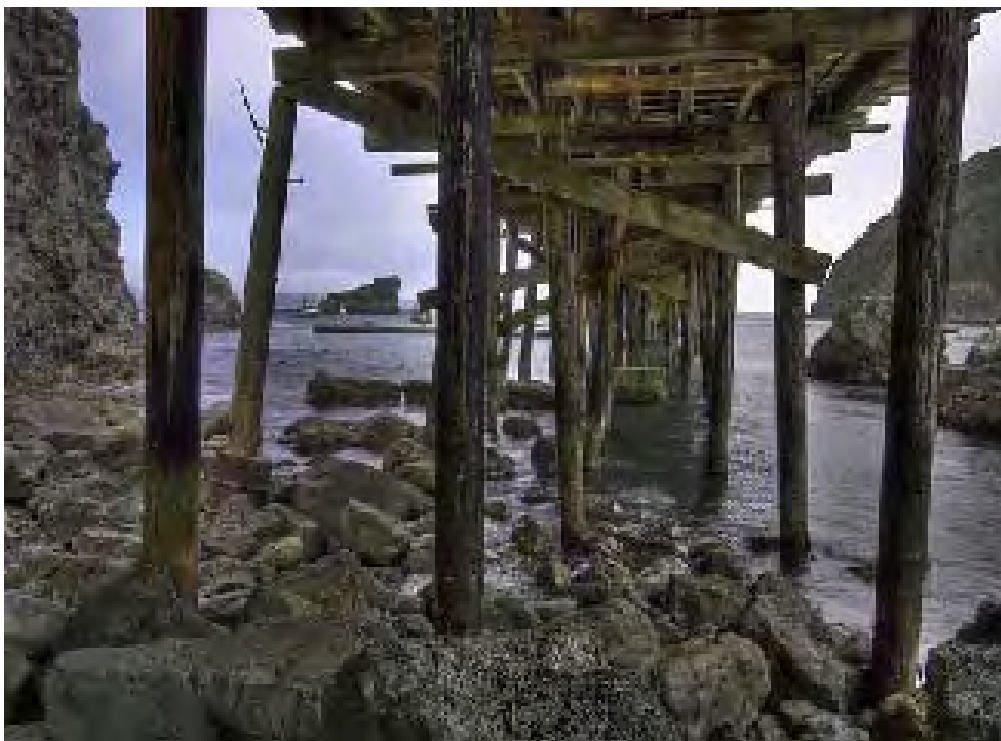
Figure 1-2. Photo showing deteriorated condition of existing pier and creosoted piles.
