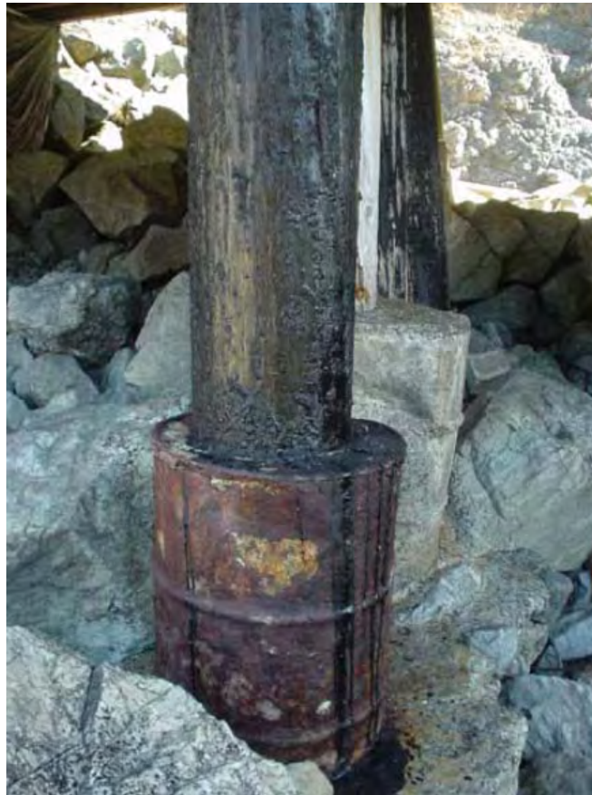
Figure 3-1. Existing pile showing creosote deposits.
