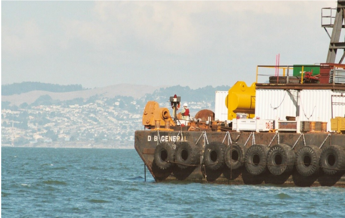
Figure 5. Example of an Observation Site (showing a marine mammal observer at the end of one of the pile driving barges)
