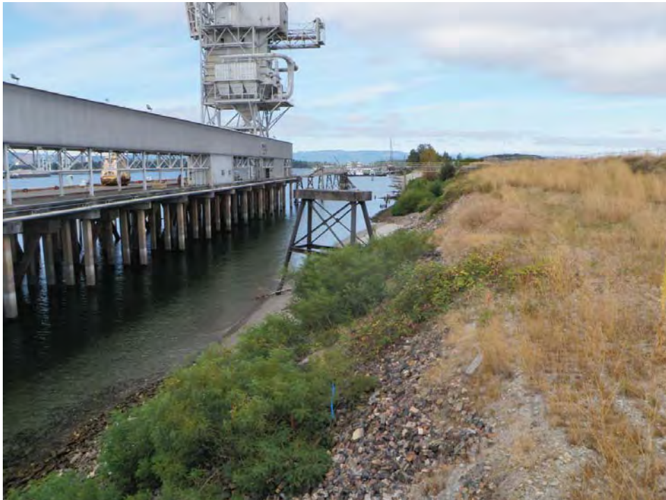
Photo 2: This photograph is taken facing west (downstream) and documents the condition of the existing dock, and the nature of the riparian and upland habitat conditions within the project area.
