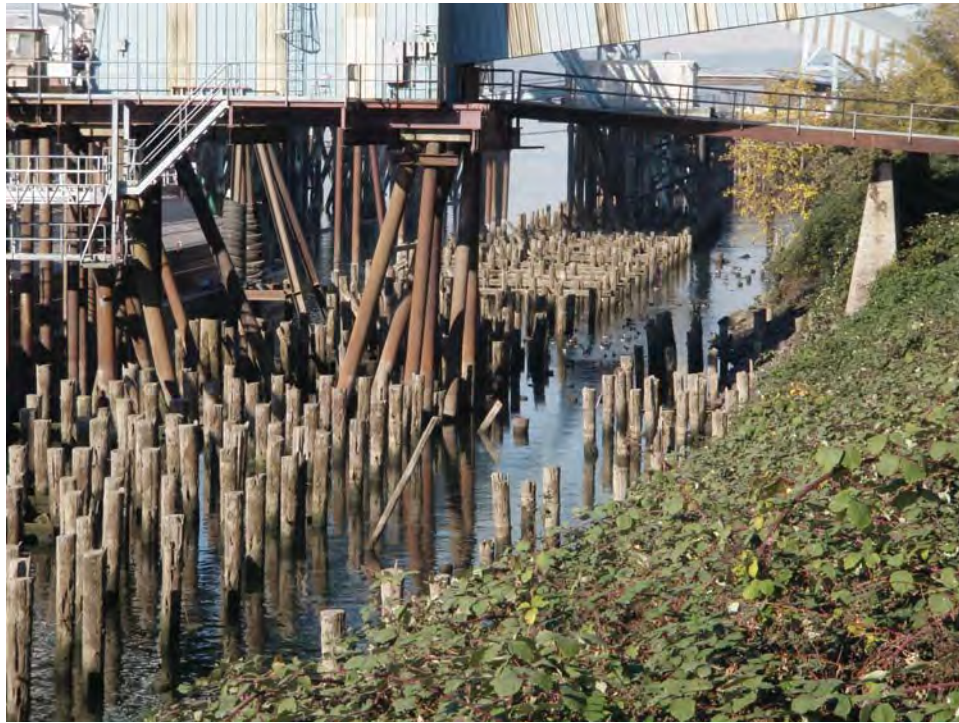
Photo 3: This photograph documents treated timber piles at Terminal 2. A portion of these piles will be removed as mitigation for the new steel piles that are required for the project.
