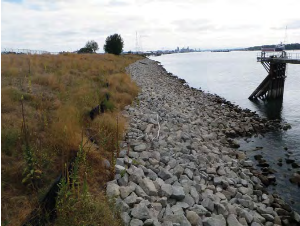
Photo 1: This photograph is taken facing east (upstream) from the existing dock, and documents the riparian and nearshore conditions at the site and the extent of bank armoring.
