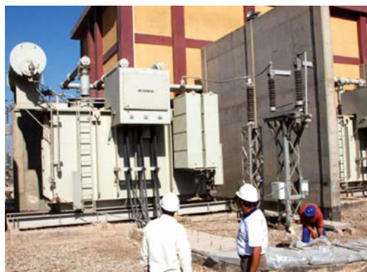
USACE completed construction of the 132-33 kV al-Farabi substation in Sadr City in February and turned it over to the MOE. (USACE photo)
