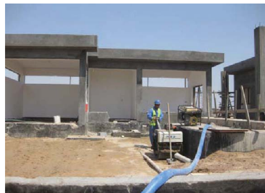
A worker on site at al-Kibla Sewer and Storm Network in Basrah province. (USACE photo)
