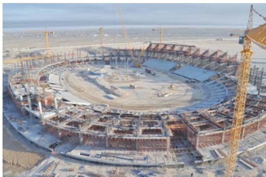
Main stadium of Basrah Sports City project under construction in early 2011. Stadium will seat 65,000 and have both a soccer field and light athletics track that conform to international standards. (Malachy Walsh and Partners photo)
