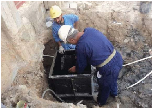
Workmen lay piping to hook up residential homes to the Falluja Waste Water Treatment System in Anbar province. (USACE photo)
