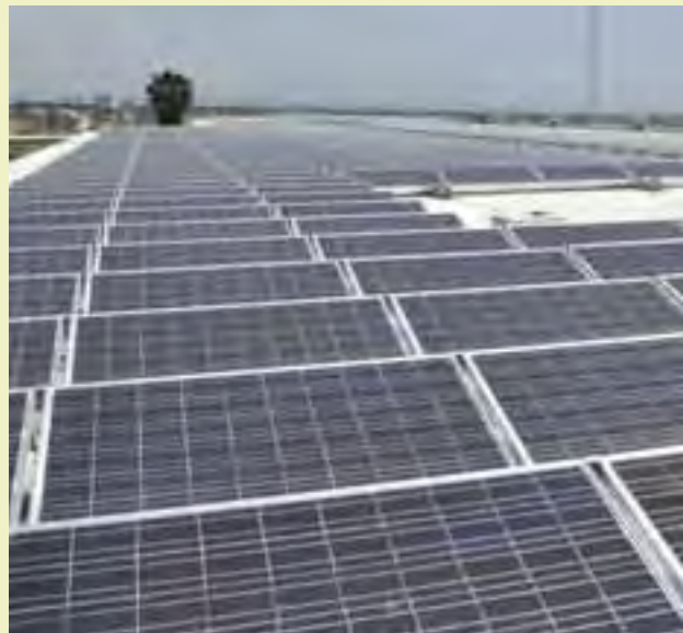
A total of almost 400 kilowatts of rooftop renewable energy photovoltaic systems went online at NWS Seal Beach in FY11. These systems have created an annual savings of over $90,000.
