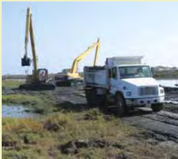
Slag and ash residue is removed from a NBVC Point Mugu lagoon. It took six weeks to remove the ash and slag residue, which totaled almost 2,000 cubic yards.
