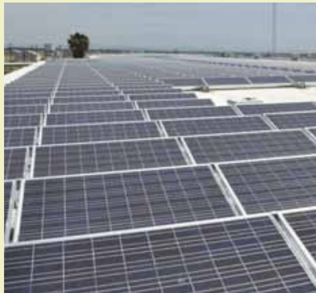
A total of almost 400 kilowatts of rooftop renewable energy photovoltaic systems went online at NWS Seal Beach in FY11. These systems have created an annual savings of over $90,000.
