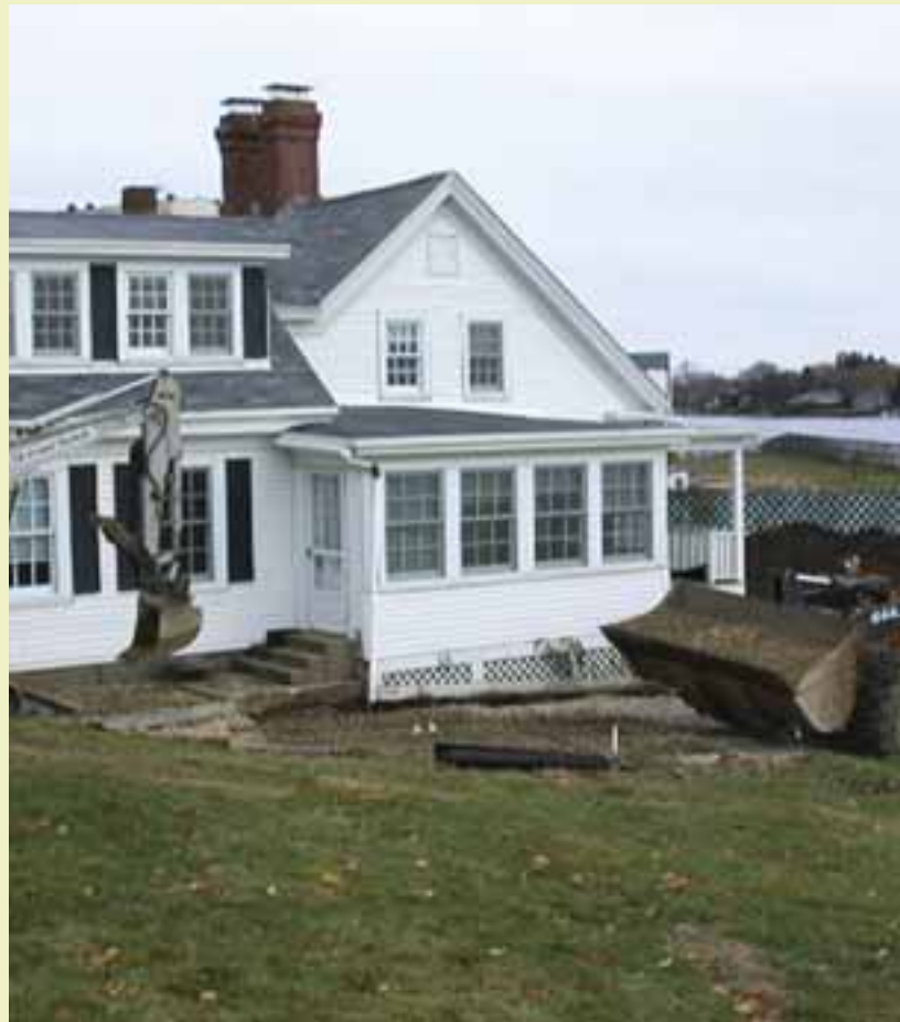
After soil sampling activities were completed at PNSY, each area was backfilled with gravel, lined with geotextile fabric, and top dressed with loam and seed. Final backfilling, landscaping, and fence replacement were completed during fall 2010 and spring 2011.
